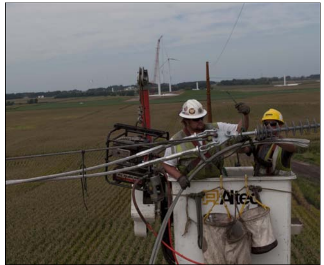
Hooper Corporation crewmembers dead end wire on steel structures and make jumper connections.
