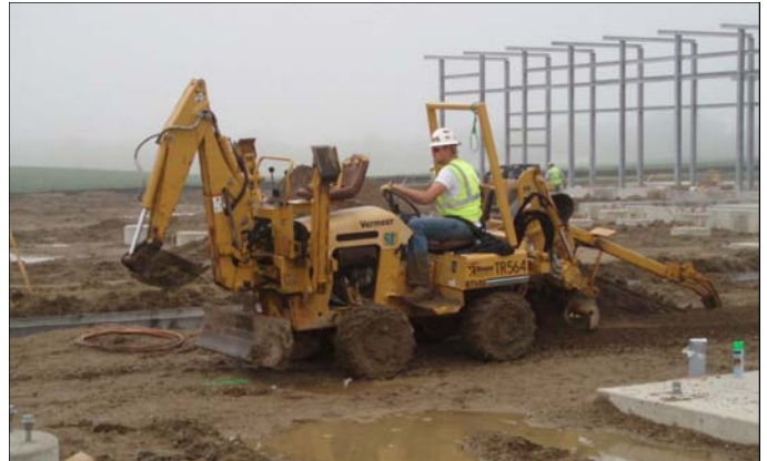
Crewmembers struggle through wet and muddy conditions to trench in the 4/0 copper ground grid.
