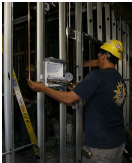
Plumbers worked nights and weekends to complete the upgrade to St. Mary's Hospital.
